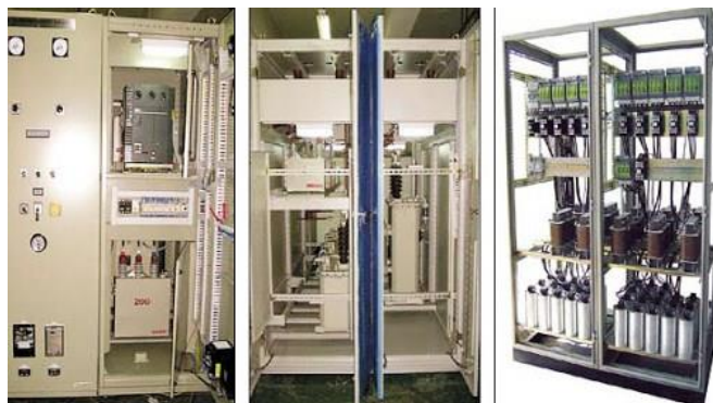
Gambar 2. 10 Kapasitor Bank Cubicle (Sumber : www.riverspace.org )
