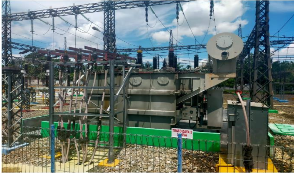
Gambar 3.3 Tranformator Daya 2 (TD 2)
