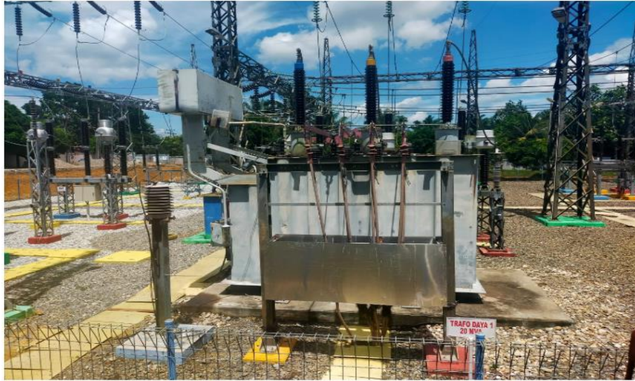
Gambar 3.2 Tranformator Daya 1 (TD 1)
