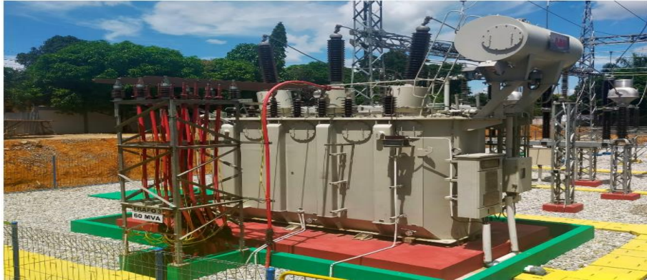
Gambar 3.4 Tranformator Daya 3 (TD 3)
